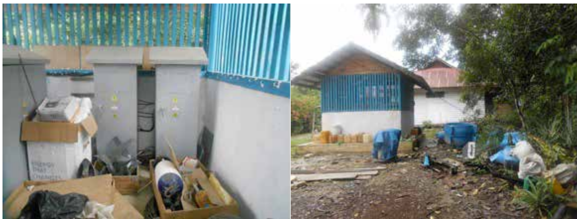
Gambar 17. The damaged pumps received from GTZ, Germany
